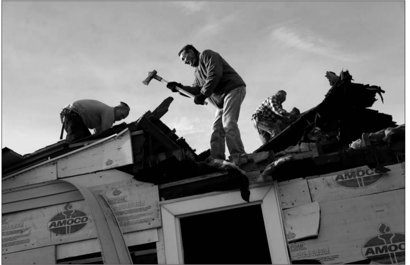
John Toto, center, works with friends to demolish his house in the Midland Beach section of Staten Island, N.Y., on Friday. About 200 homes damaged by Hurricane Sandy will be bulldozed in the coming days.
